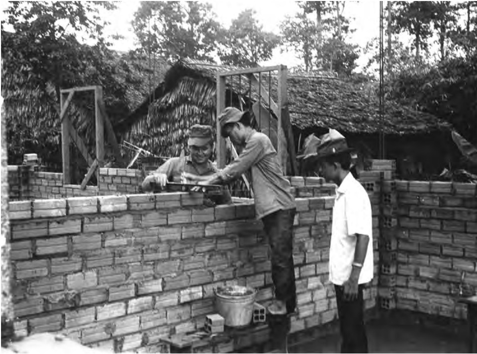
Beginning in 1963, teams of Army and Navy engineers carried out building projects such as this dispensary by the Seabees.
